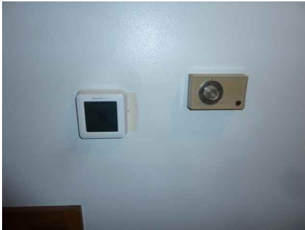
Programmable Thermostat and Humidistat in Main Hallway
