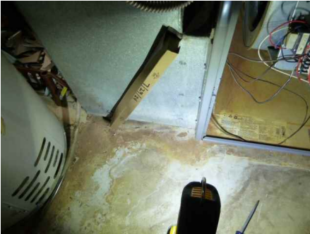
Water stains on floor and inside furnace cabinet. Past humidifier leak possible
