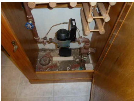
Water shut off and sewer cleanout in basement across from stairs in cabinet
