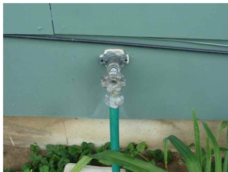
Rear spigot leaks when opened. Needs repair
