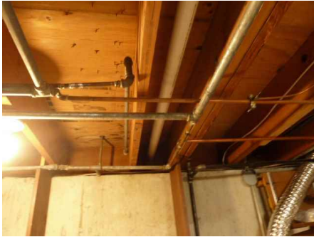
Copper and galvanized water supply connections incorrect. Corrosion probable
