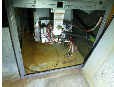
Water stains inside furnace cabinet. Monitor humidifier filter
