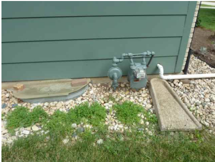
Gas meter located at southeast corner of structure
