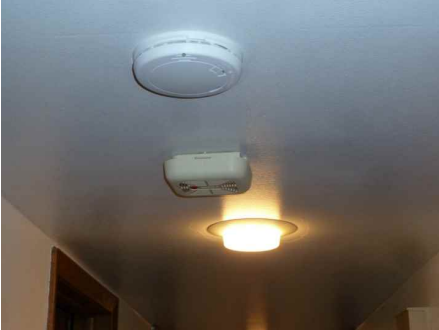
Smoke Alarms in main hall near bedrooms
