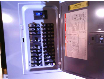
Incomplete panel labeling
