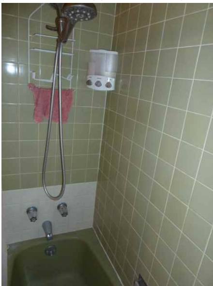
Missing drain stopper. Previous faucet replacement assumed by ceramic tile patch
