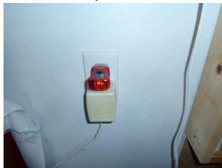
Garage receptacle not properly grounded and no GFCI. Correction needed
