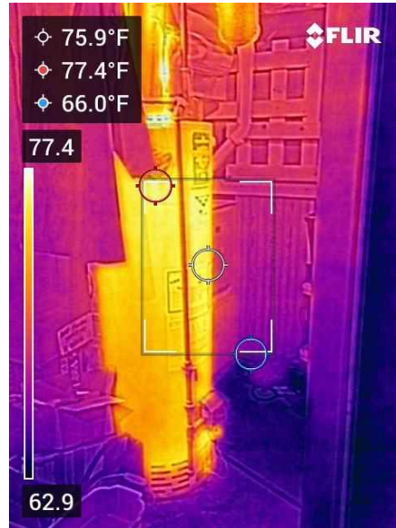
Thermal image of water heater operating
