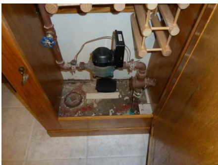
Water shut off and sewer cleanout in basement across from stairs in cabinet
