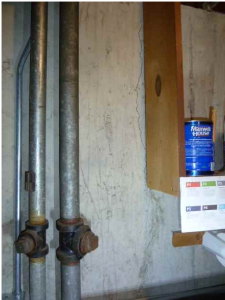
Small crack in foundation at west wall. Monitor for changes or moisture penetration
