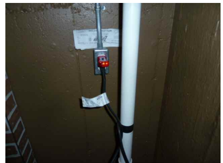
Sump pump receptacle properly grounded but should have GFCI protection
