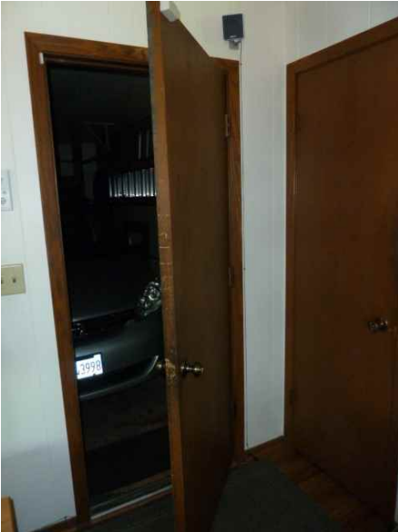
No self-closer on entry door to interior of home
