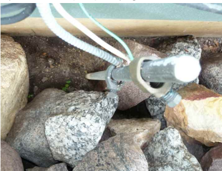
Two ground wires under one nut not correct
