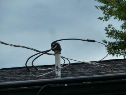
Overhead service weather head too low for proper drip loop height
