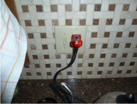
Properly wired GFCI outlet at kitchen sink area
