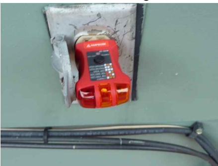
Rear deck receptacle not grounded and no GFCI installed. Safety issue. Correction needed
