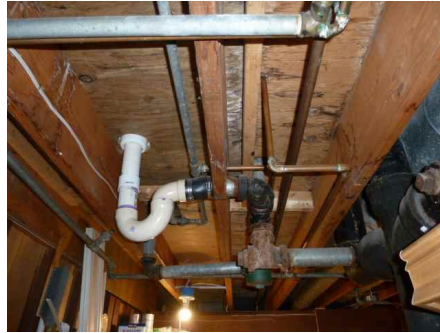
Water supply connections incorrect. Recommend repair or replacement
