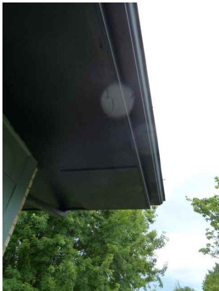
Small plywood patch at corner of soffit
