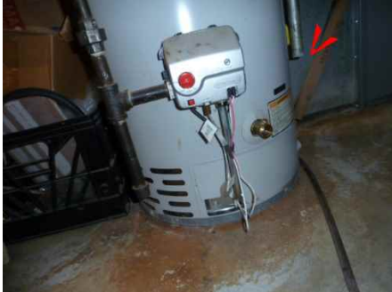
Overflow tube from pressure relief valve too short. Safety issue
