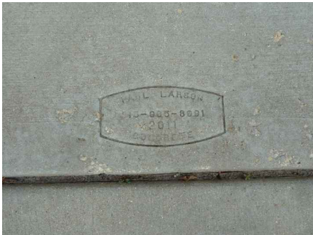
Concrete drive and sidewalk installed in 2011. Minor spalling due to salt use
