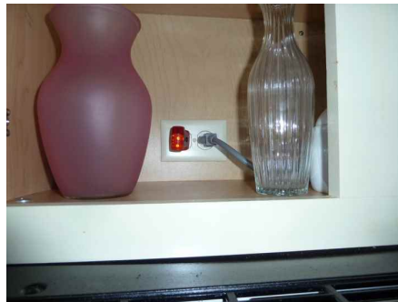
Microwave outlet properly grounded
