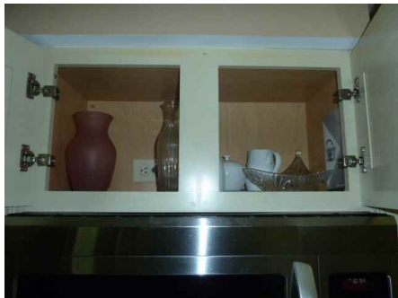
No kitchen ventilation to the outside
