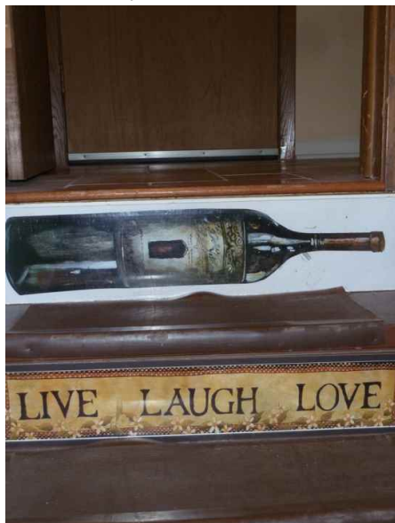
Top riser higher due to floor upgrade in kitchen. Possible trip hazard
