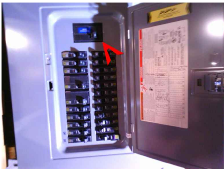
Main Electrical Disconnect at west wall in basement laundry area
