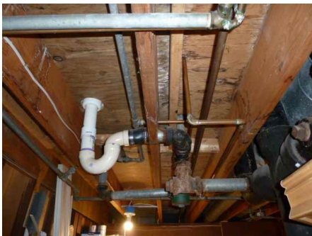
Staining under bathroom area. Monitor for leaks
