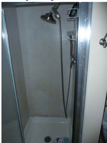
Reseal wall to shower base connection
