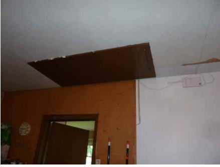
Attic access in garage is a fire safety concern.
