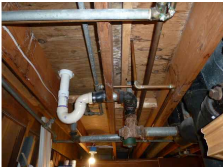
Stains on subfloor. Monitor for leaks
