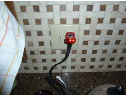
GFCI protected receptacle near kitchen sink area
