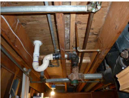
Notched joist where drain passes through it. Monitor and repair if needed
