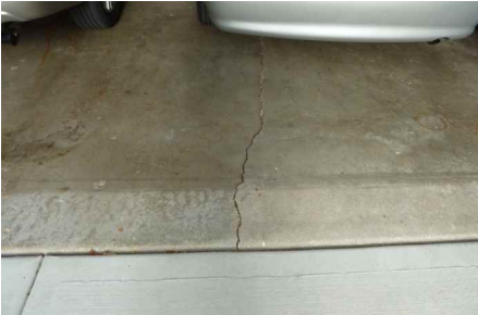
Cracks in garage floor due to settling. Monitor for changes
